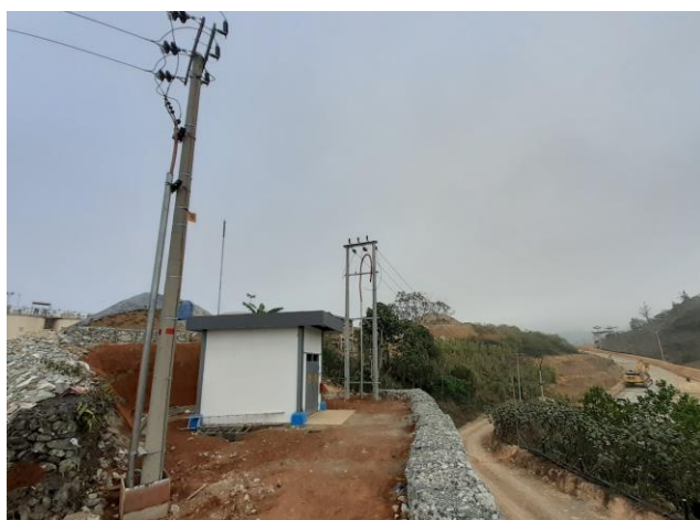
Figure 1: New Transformer building – Way Linggo
